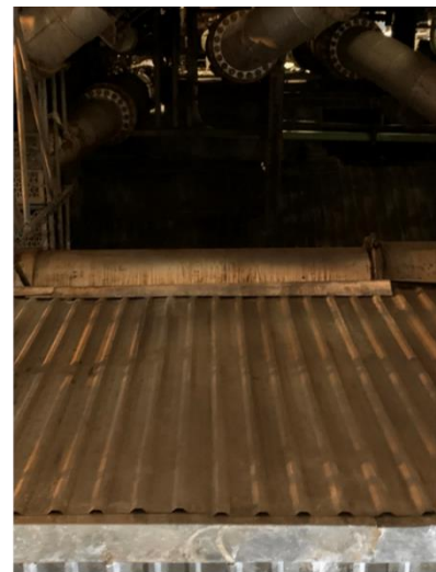
An incinerator suspended above our heads
